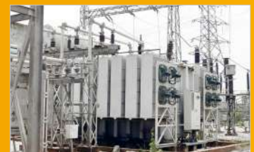
2x20/25MVA, 110/11.5kV Power Transformers Dangote Cement, Congo
