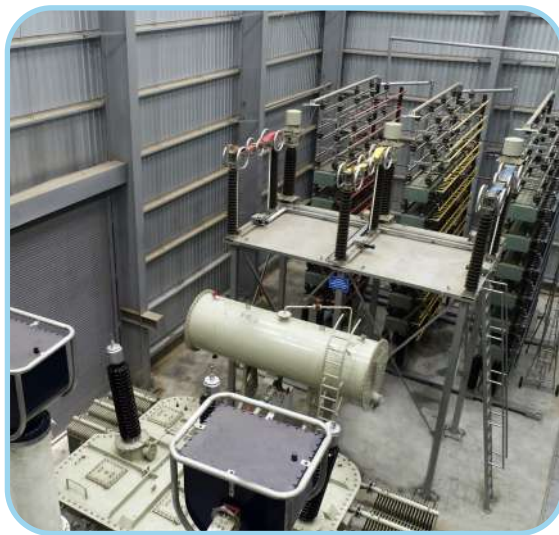
State-of-the-Art UHV Transformer Test Laboratory
