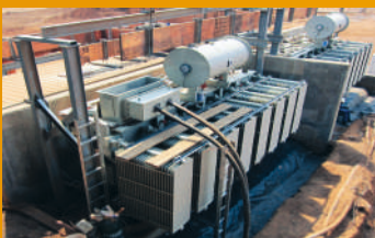
2x(4005/2823-2823)kVA, 33kV, 2x565V 12 Pulse Rectifier Transformer in South Africa
