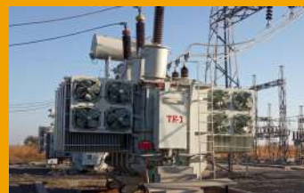
40/50MVA, 132/33kV Power Transformer, ReGen Powertech, Rajasthan, India
