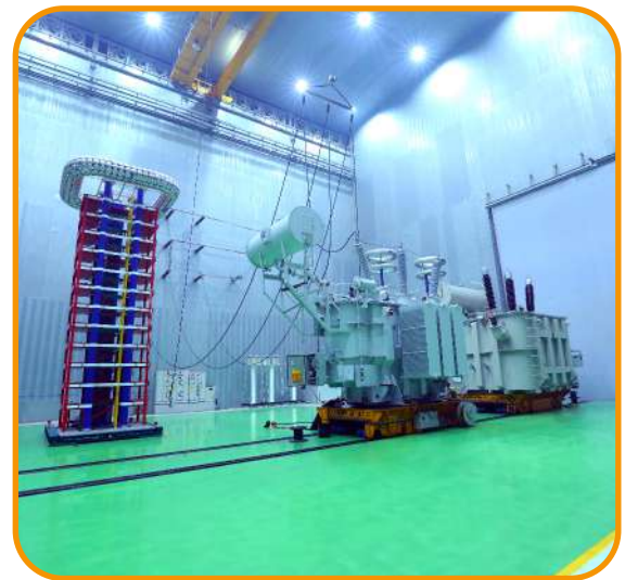
2400KVP, 360k J (Expandable) Impulse Generator and 6 Channels Partial Discharge Testing Facility
