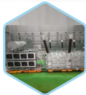
500MVA, 400kV Transformer Testing
