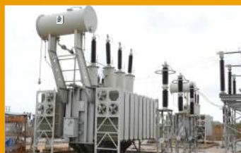
2x60MVA, 132/33kV Power Transformers installed at Kudendan Power Plant in Kaduna, Nigeria
