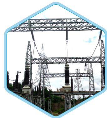
132kV CTs & PTs Lafarge Cement, Ogun State, Nigeria
