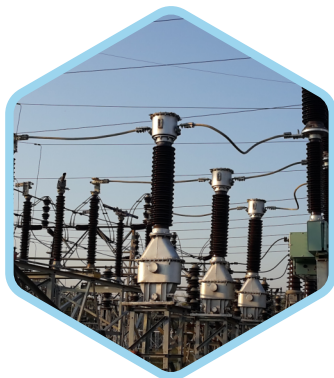
132kV CTs & PTs TI Steels, Himachal Pradesh, India
