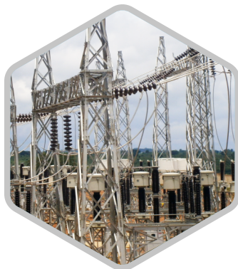
132kV CTs & PTs TCN, Kaduna, Nigeria
